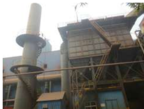
1#高炉矿槽上料废气布袋除尘器+排气筒
